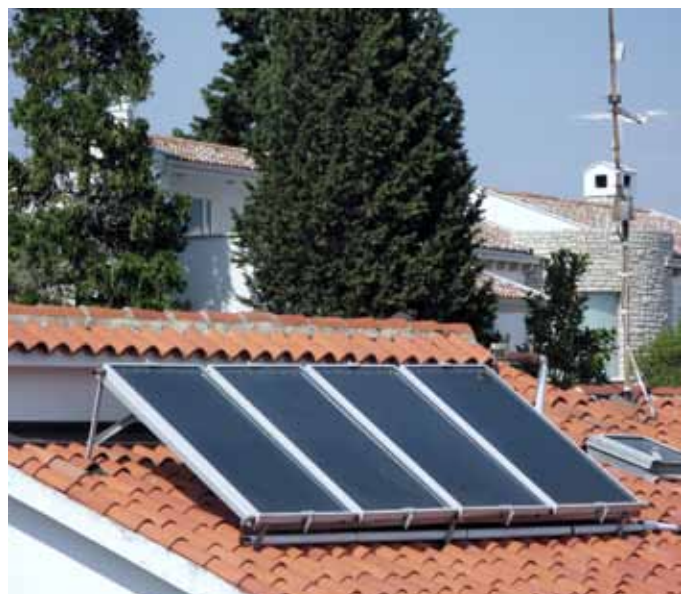
Illustration 4. Solar water heaters on a roof
