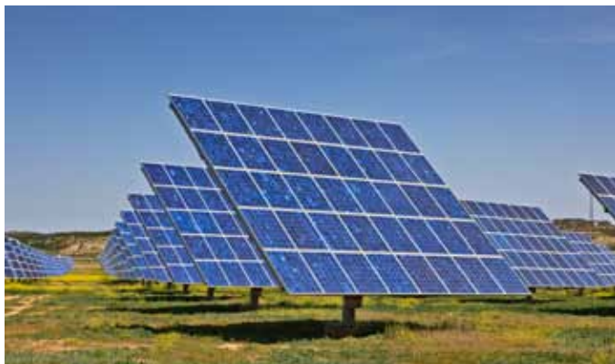
Illustration 7. A solar array
